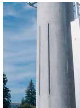
Toothed anchor channels in concrete masts for fixing the most equipment.
