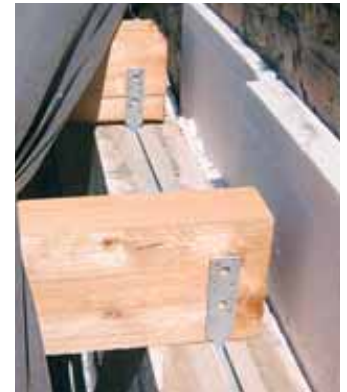
Joist fixing to ring beam with nail ties and brick tie channels
